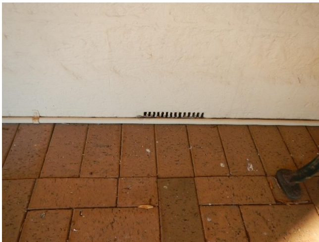
Substantially covered sub floor vent.
