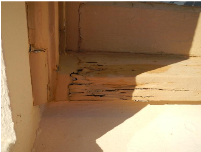
Rotted window sills and window frame
