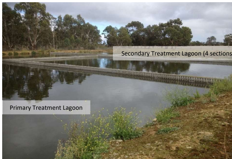
Figure 6 Treatment Lagoon at Kalangadoo
