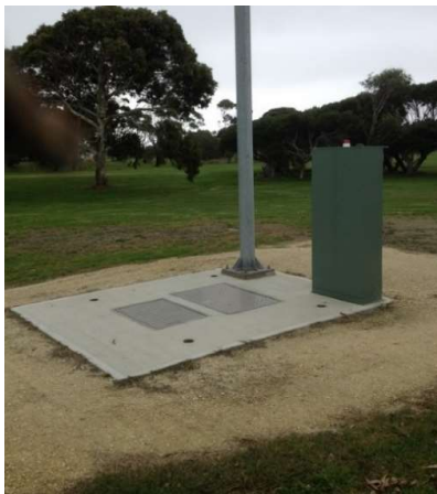
Figure 11 Pump Station 4 adjacent Beachport Visitor Information Centre
