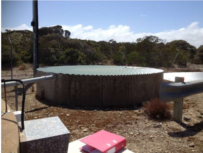
Figure 8 Sludge thickening tank at Southend WWTP
