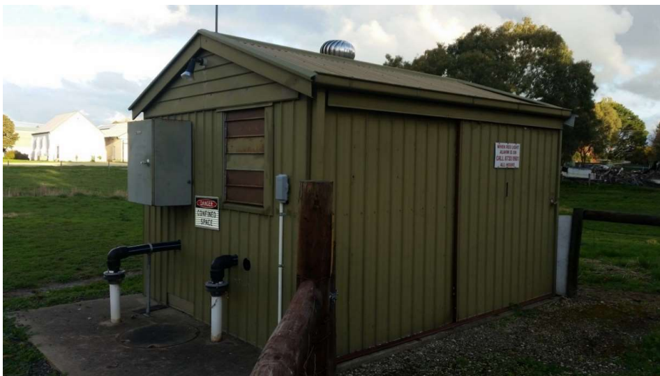
Figure 5 Pump Station 1 at Kalangadoo
