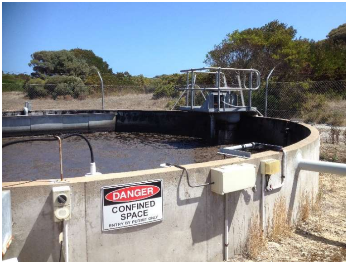
Figure 7 Intermittent aerator at Southend Wastewater Treatment Plant (WWTP)
