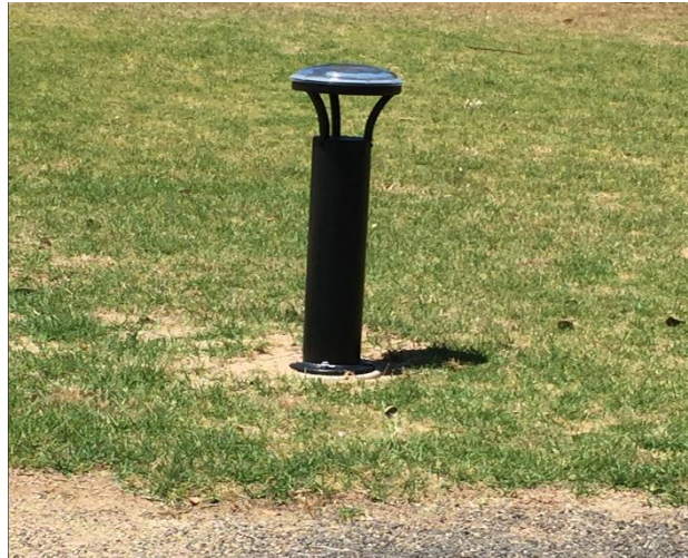
Footpath bollard light
